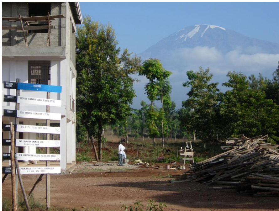
The construction site of the Kilimanjaro Clinical Research Centre at the foot of Mount Kilimanjaro
